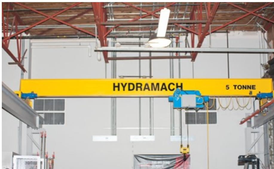
Figure 48 Overhead travelling crane (BC Industry Training Authority, 2019). CC BY-NC-SA 4.0 ( https://creativecommons.org/licenses/by-nc-sa/4.0/ )
