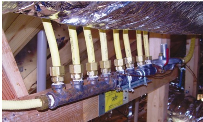
Figure 113 CSST installation, manifold and support bracket and regulator (BC Industry Training Authority, 2019). CC BY-NC-SA 4.0 ( https://creativecommons.org/licenses/by-nc-sa/4.0/ )
