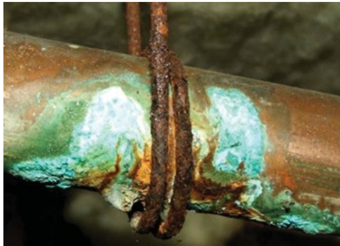
Figure 51 Stray current accelerating corrosion of a copper pipe
