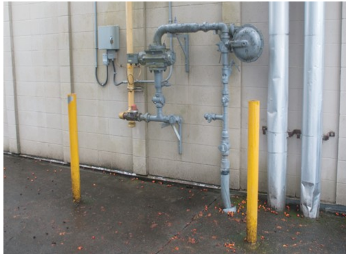
Figure 63 Pipe bollards filled with concrete and placed to prevent vehicle damage to the gas service entry and meter located in a driveway. (BC Industry Training Authority, 2019). CC BY-NC-SA 4.0 ( https://creativecommons.org/licenses/by-nc-sa/4.0/ )
