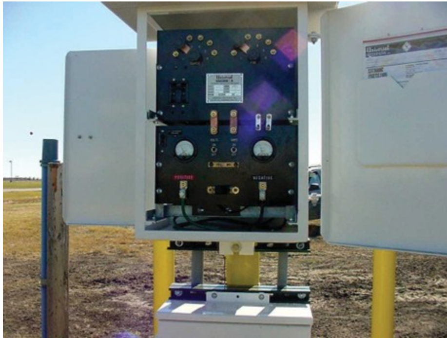
Figure 43 An air-cooled cathode protection rectifier connected to a pipeline (BC Industry Training Authority, 2019). CC BY-NC-SA 4.0 ( https://creativecommons.org/licenses/by-nc-sa/4.0/ )
