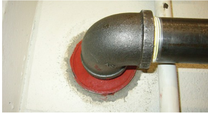
Figure 51 Fire stop in concrete (BC Industry Training Authority, 2019). CC BY-NC-SA 4.0 ( https://creativecommons.org/licenses/by-nc-sa/4.0/ )
