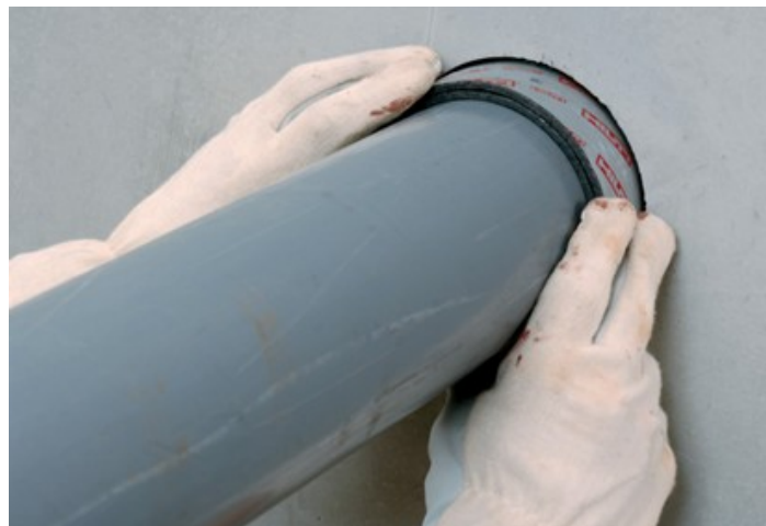
Figure 9 Firestop wrap (BC Industry Training Authority, 2019). CC BY-NC-SA 4.0 ( https://creativecommons.org/licenses/by-nc-sa/4.0/ )
