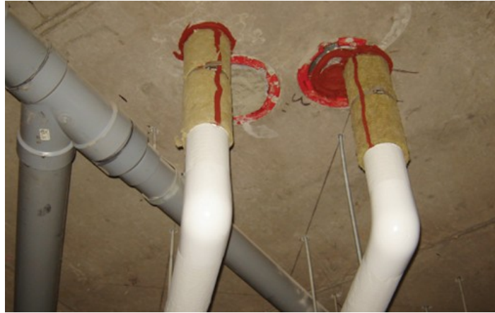
Figure 55 Insulated water pipe passing through the underside of a concrete slab in an underground parking lot (BC Industry Training Authority, 2019). CC BY-NC-SA 4.0 ( https://creativecommons.org/licenses/by-nc-sa/4.0/ )
