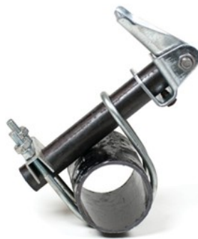
Figure 50 U-clamp on a pipe and sway brace pipe and attachment assembly (BC Industry Training Authority, 2019). CC BY-NC-SA 4.0 ( https://creativecommons.org/licenses/by-nc-sa/4.0/ )
