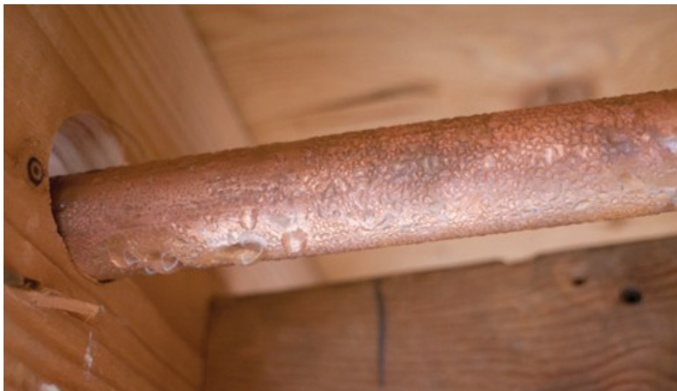
Figure 14 Condensation on a pipe (BC Industry Training Authority, 2019). CC BY-NC-SA 4.0 ( https://creativecommons.org/licenses/by-nc-sa/4.0/ )
