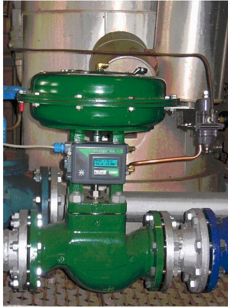
Figure 4 PI control valve ( https://commons.wikimedia.org/wiki/File:PI_control_valve.jpg ) (Rafał Rygielski/ Wikimedia Commons)
