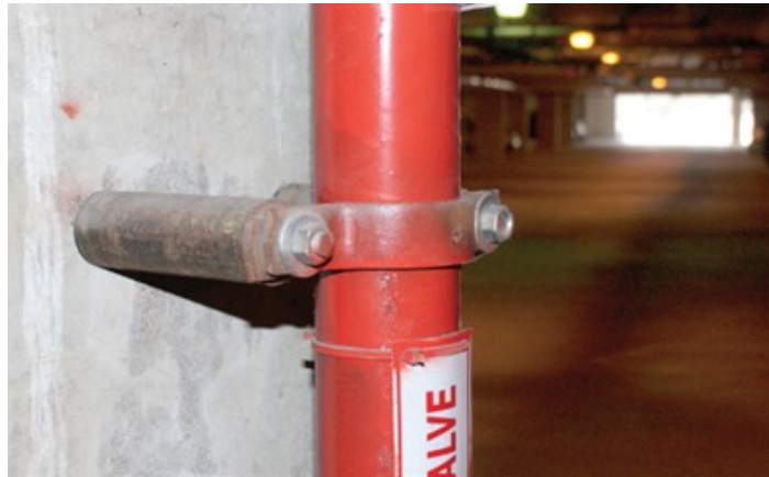
Figure 43 Riser clamp on pipe attached to concrete wall structure (BC Industry Training Authority, 2019). CC BY-NC-SA 4.0 ( https://creativecommons.org/licenses/by-nc-sa/4.0/ )
