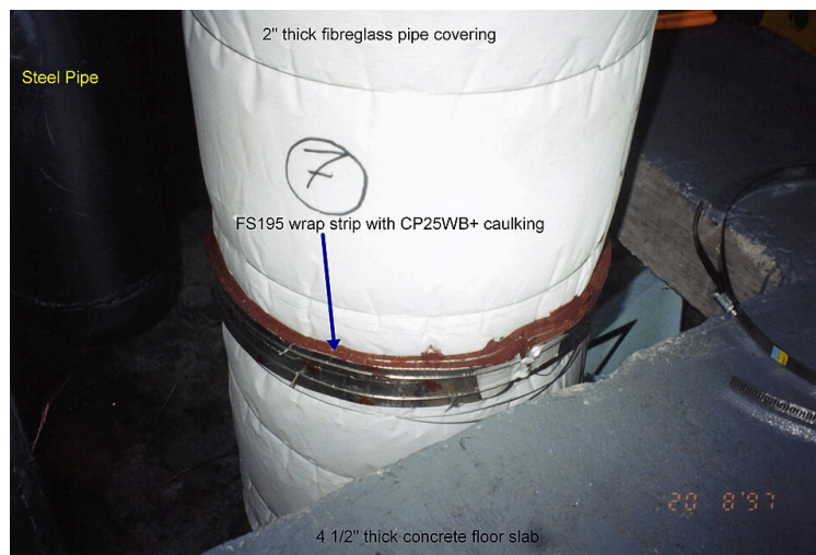
Figure 56 Fiberglass pipe covering ( https://commons.wikimedia.org/wiki/File:Fs195_cp25_fibreglass_pc.jpg ) by Achim Hering ( https://commons.wikimedia.org/wiki/User:Achim_Hering ) from Wikimedia Commons
