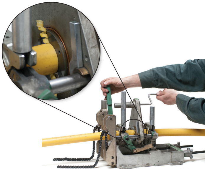
Figure 72 Facing the pipe end (BC Industry Training Authority, 2019). CC BY-NC-SA 4.0 ( https://creativecommons.org/licenses/by-nc-sa/4.0/ )
