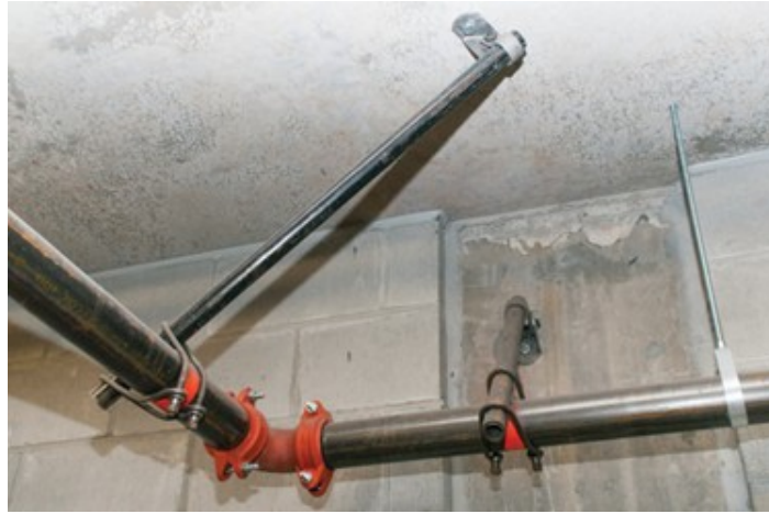
Figure 52 Sway brace on a fire sprinkler system (BC Industry Training Authority, 2019). CC BY-NC-SA 4.0 ( https://creativecommons.org/licenses/by-nc-sa/4.0/ )
