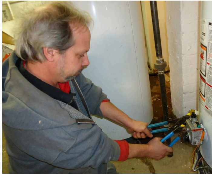
Figure 92 Wrenches to tighten a fitting ( https://commons.wikimedia.org/wiki/File:Plumber_uses_two_wrenches_to_tighten_a_fitting.jpg ) (Tomwsulcer/Wikimedia Commons) CC0 1.0 ( https://creativecommons.org/publicdomain/zero/1.0/deed.en )
