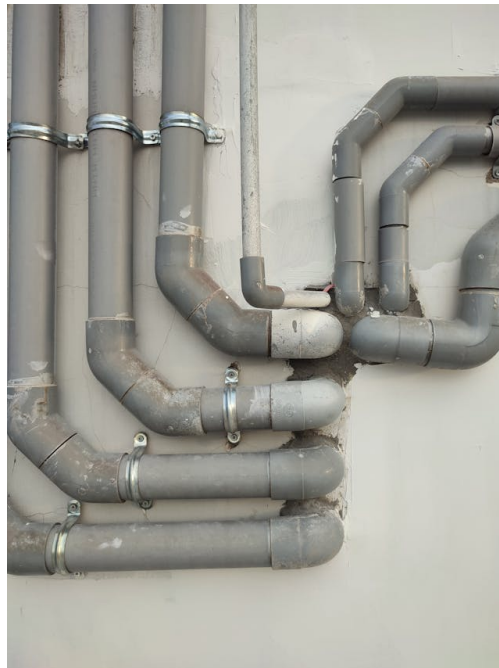
Figure 88 Plastic Pipes joint ( https://www.pexels.com/photo/plastic-pipes-on-wall-12142829/ ) (Bùi Hoàng Long/Pexels) Pexels license ( https://www.pexels.com/license/ ).
