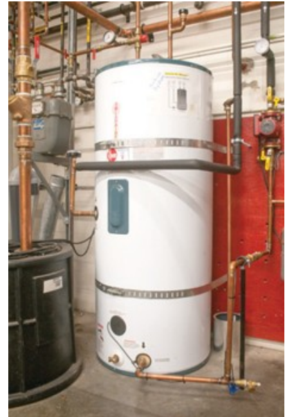
Figure 59 Hot water storage heater with seismic restraint using manufactured strapping (BC Industry Training Authority, 2019). CC BY-NC-SA 4.0 ( https://creativecommons.org/licenses/by-nc-sa/4.0/ )
