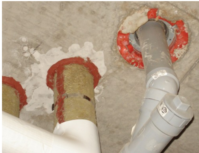
Figure 52 Firestop in parking garage ceiling (BC Industry Training Authority, 2019). CC BY-NC-SA 4.0 ( https://creativecommons.org/licenses/by-nc-sa/4.0/ )
