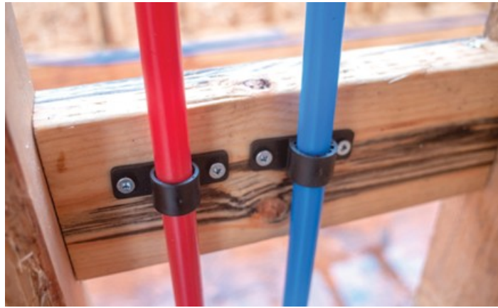
Figure 61 Residential application of pipe clips used to support and hold PEX tubing (BC Industry Training Authority, 2019). CC BY-NC-SA 4.0 ( https://creativecommons.org/licenses/by-nc-sa/4.0/ )
