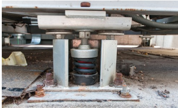
Figure 40 Spring isolator supports under an outdoor refrigeration condenser unit (BC Industry Training Authority, 2019). CC BY-NC-SA 4.0 ( https://creativecommons.org/licenses/by-nc-sa/4.0/ )
