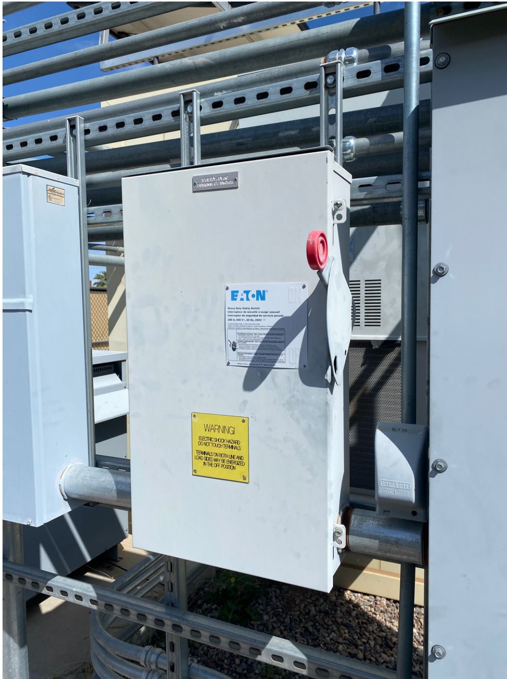
Figure 15 A utility disconnect switch to control power to a building. It controls 3-phase 120/208 V, 200A service to a commercial building. (Rsparks3/Wikimedia Commons) CC0 1.0
