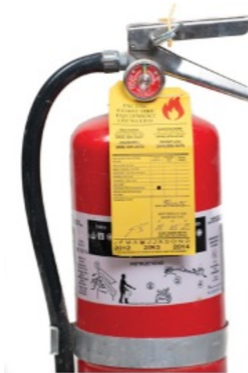
Figure 6 ABC fire extinguisher with inspection tag (BC Industry Training Authority, 2019). CC BY-NC-SA 4.0 ( https://creativecommons.org/licenses/by-nc-sa/4.0/ )
