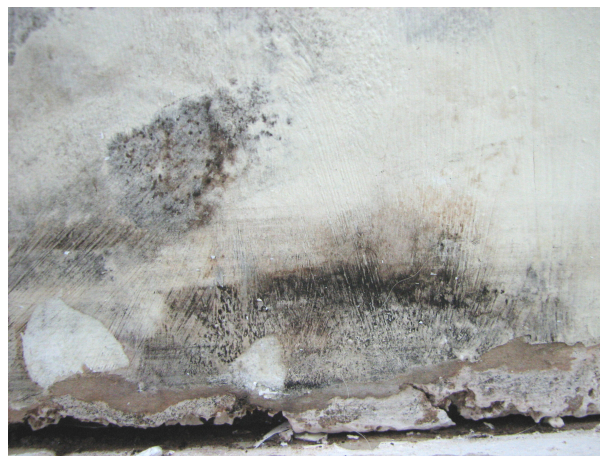
Mould on concrete wall (fdplipe/FreeImages) Freeimages.com Content License ( https://www.freeimages.com/license )
