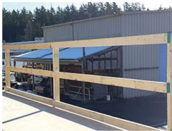
Figure 12 Guardrail and midrail—close up. (BC Industry Training Authority, 2019). CC BY-NC-SA 4.0 ( https://creativecommons.org/licenses/by-nc-sa/4.0/ )
