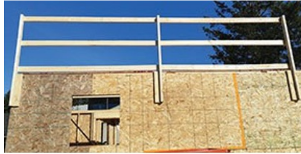
Figure 11 Guardrail and midrail (BC Industry Training Authority, 2019). CC BY-NC-SA 4.0 ( https://creativecommons.org/licenses/by-nc-sa/4.0/ )
